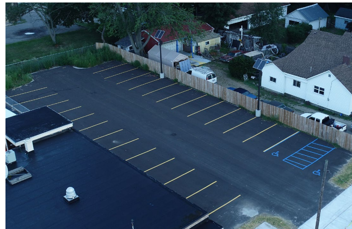
Vicksburg Michigan, USA Parking Lot Lighting Project
